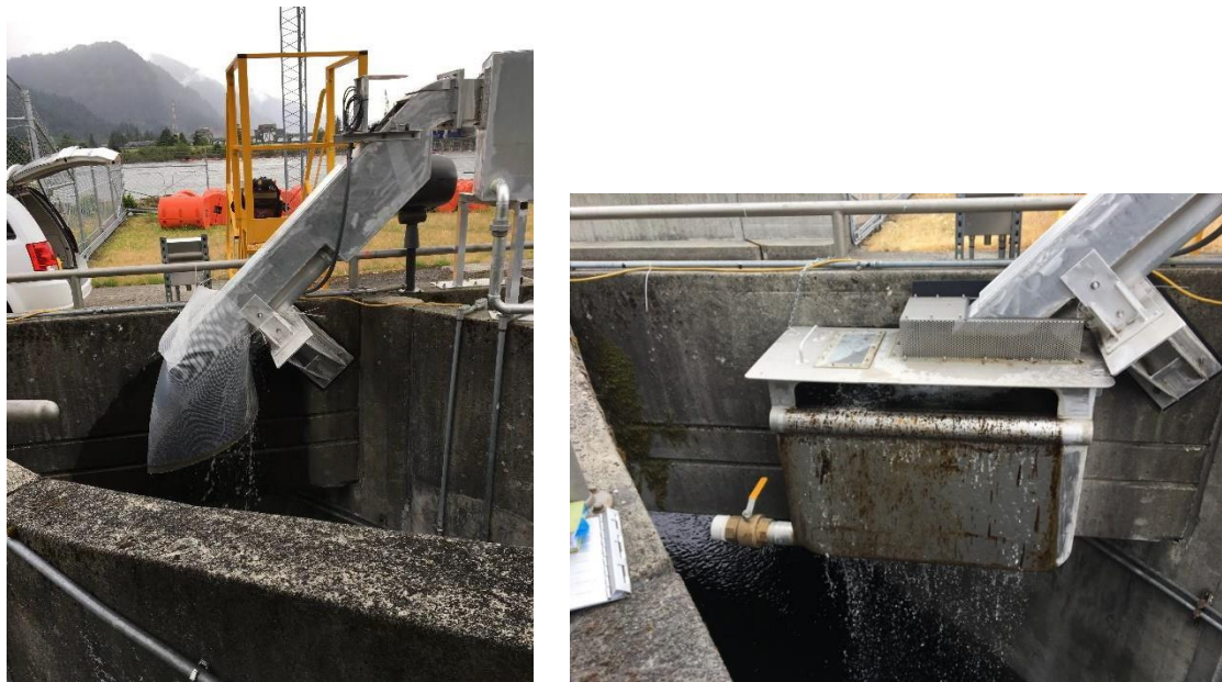
Figure 8. At the WA-AWS exit a cone of fish screen material was used to prevent lamprey from grazing the bridge wall or the opposing fishway wall (left image 2017). In 2018 this was replaced with a plunge box with a rolled lip that reduced the energy of the falling lamprey and allowed them to volitionally exit (right image).
